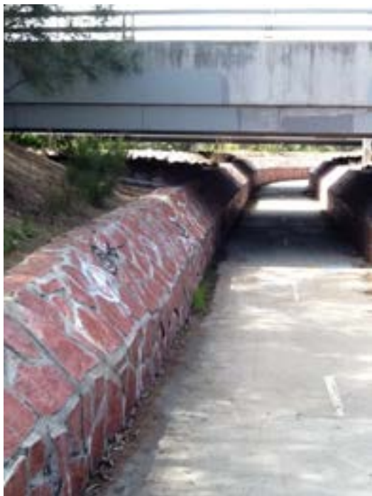
Figure 12.5: Example of Underpass Flood Mitigation, Five Islands Road, Teralba, Lake Macquarie
