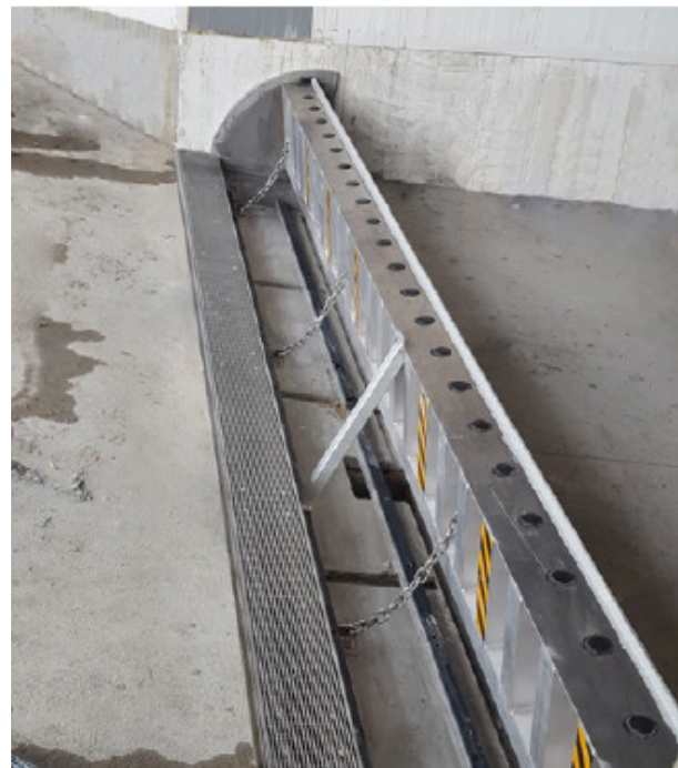
Figure 67. A self-actuating tilting flood barrier protects the entrance to a basement.
