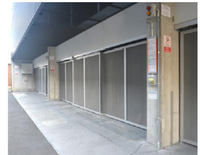
Figure 68. Self-actuating vertical-rise flood barriers South Melbourne lane.
