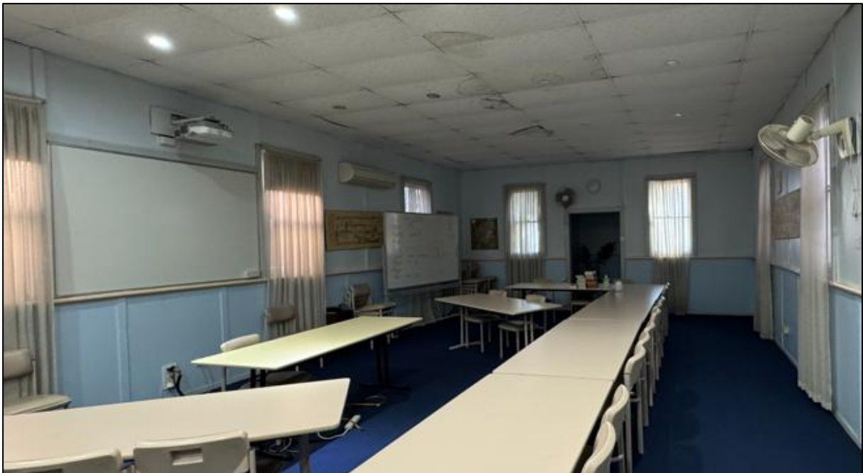
Figure 52: View of the former hall space, showing signs of water damage in the ceiling.
