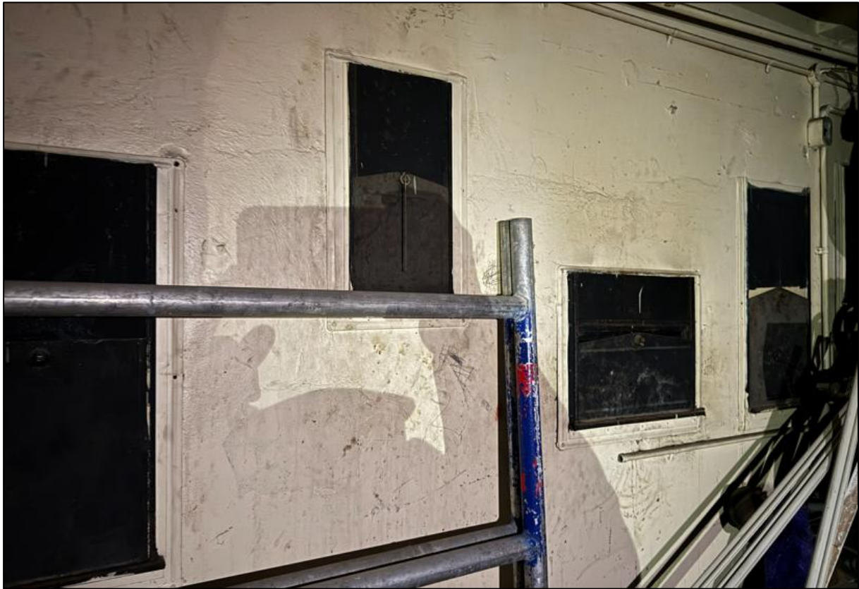
Figure 70: View of former cinema openings on northern wall of the former gallery room.
