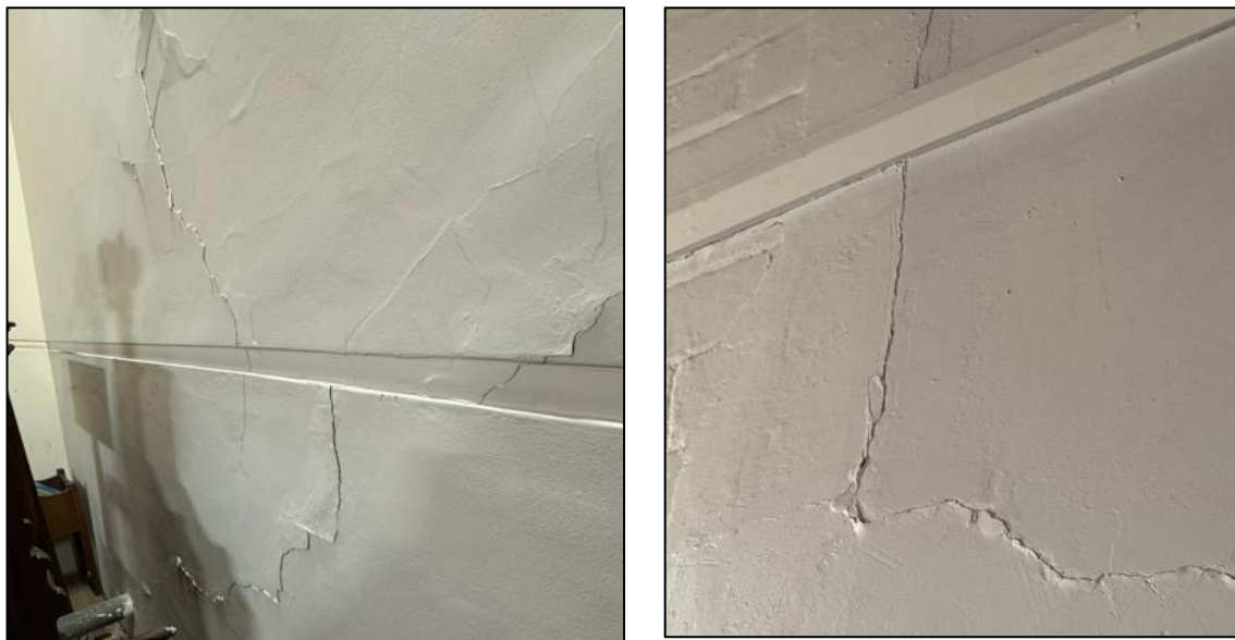
Figure 55: View of structural cracking appearing in altar and transept areas of the building.
