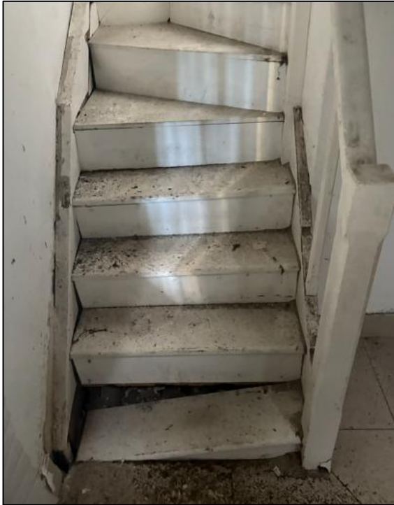
Figure 42: View of staircase leading to No. 341A first floor. It was assessed as unsafe to traverse during the inspection.
