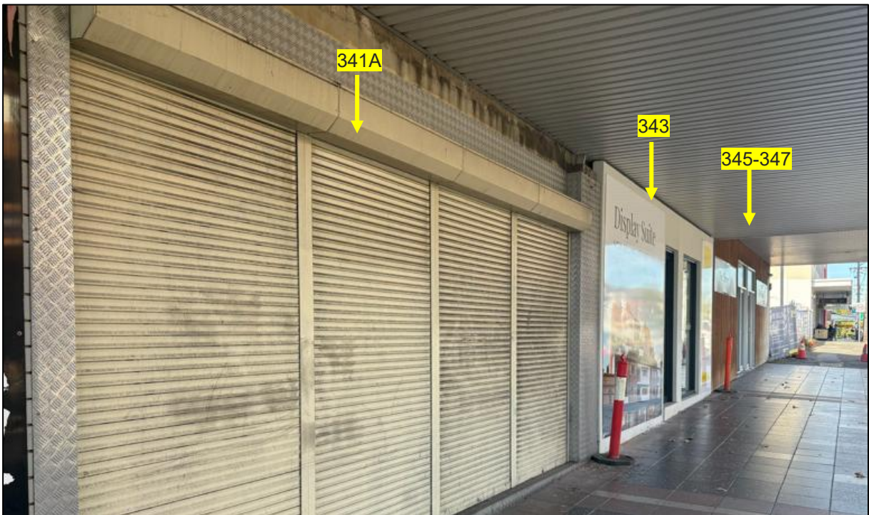
Figure 31: View of the modified shopfronts of Nos. 341A, 343 & 345-347 at the ground floor level.
